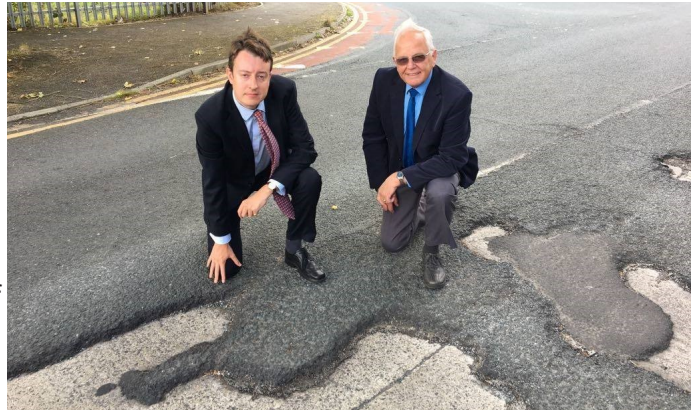
Pictured: Simon Clarke MP and Cllr Cliff Foggo by some of the damaged road surfaces.
